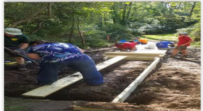
Jacob Hubbard built a boardwalk on the new section of black trail at WRNP (shown above) and installed benches at the parking lot.
